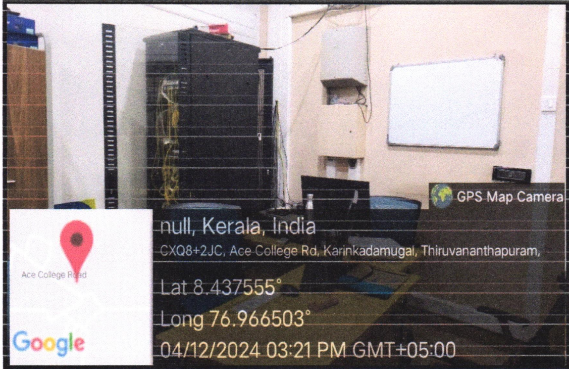
SERVER ROOM INSIDE VIEW
